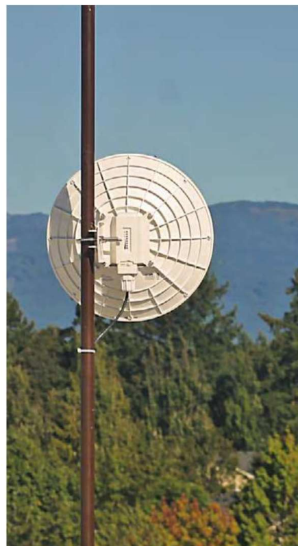
This HamWAN dish was installed at the Washington State Department of Transportation (WSDOT) in Vancouver, Washington. It's aimed at Larch Mountain. [Steve Aberle, WA7PTM, photo]
